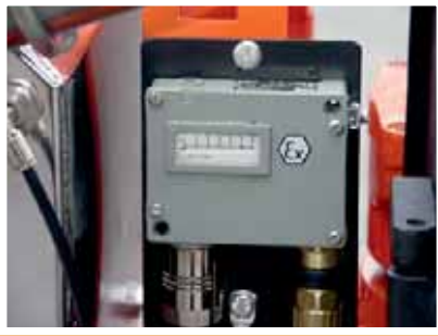
Ex Shut down pressure switch.
